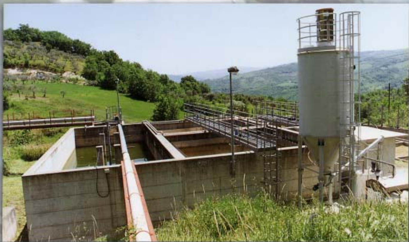
IMPIANTO BIOLOGICO PER SCARICHI CIVILI BIOLOGICAL PLANT FOR CIVIL WASTEWATER
