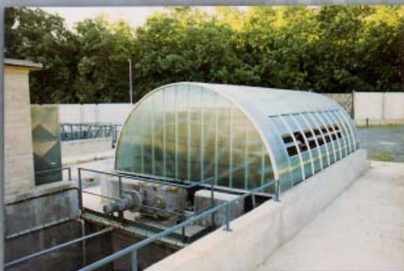
IMPIANTO BIOLOGICO PER SCARICHI CIVILI BIOLOGICAL PLANT FOR CIVIL WASTEWATER
